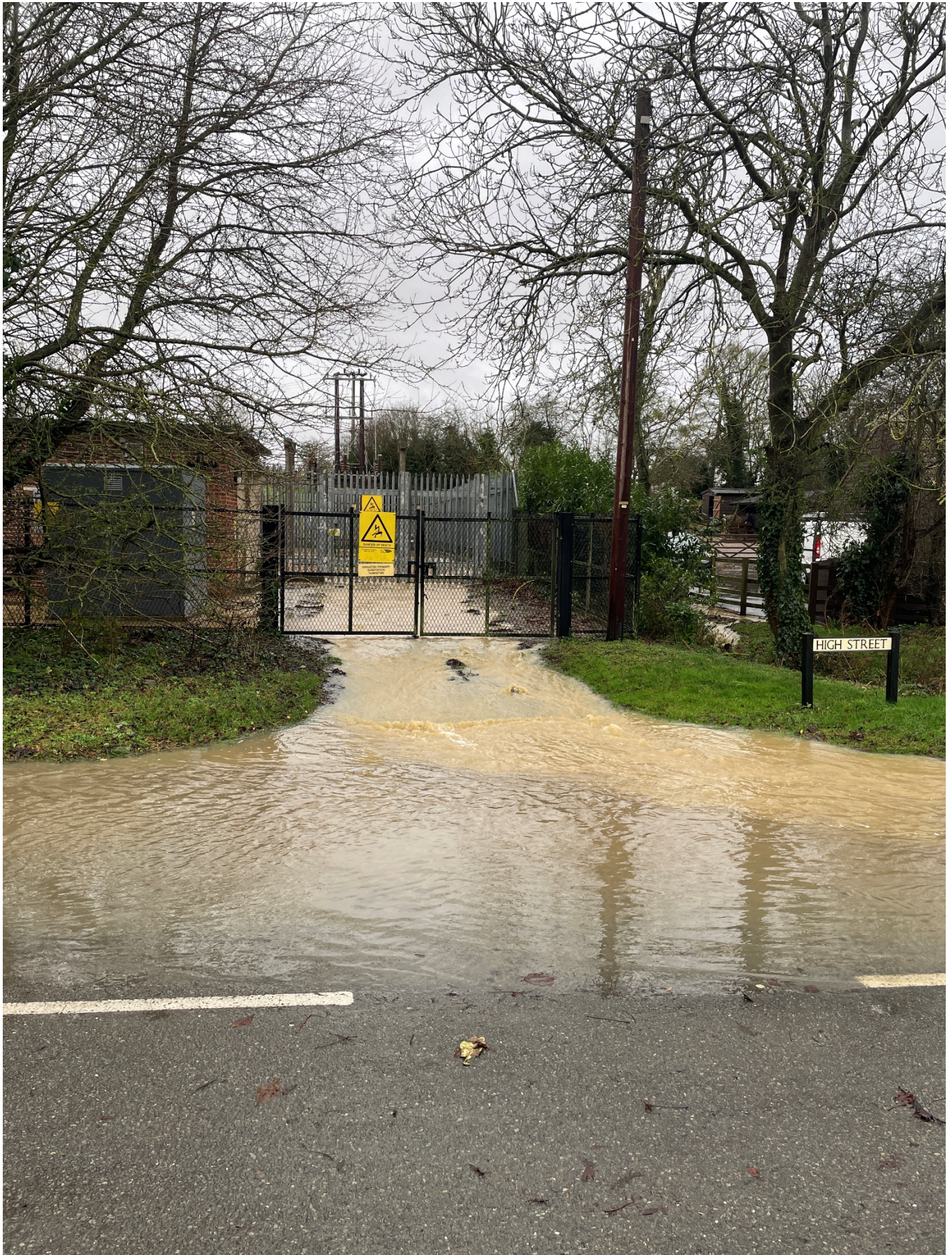
Brington Electric Sub-Station – 2 nd January 2024
